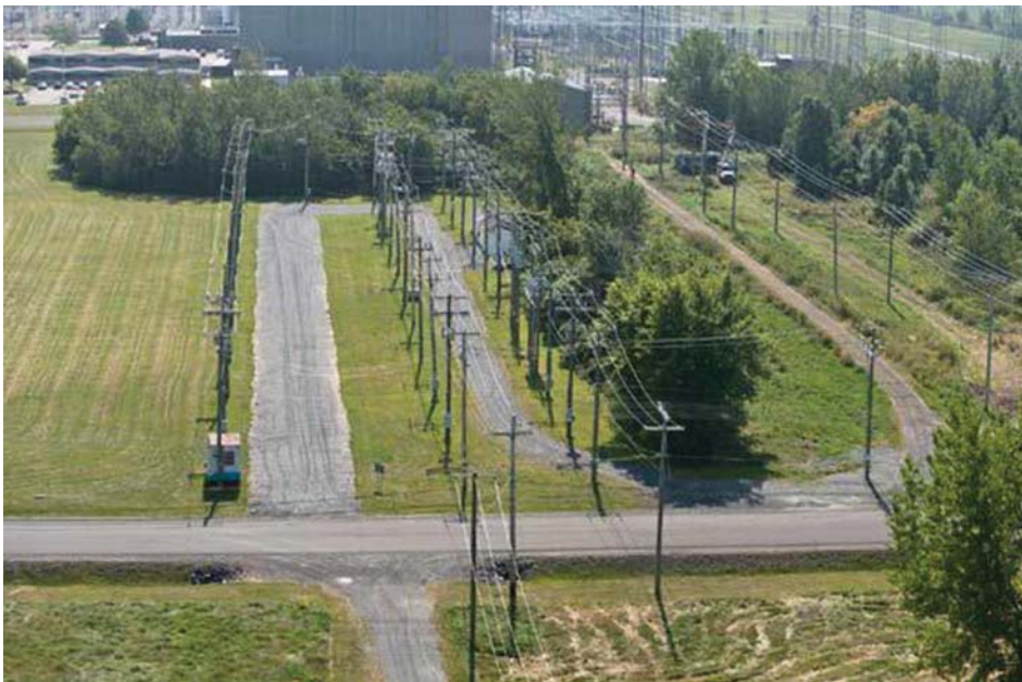
Figure 2.5 Aerial photograph of the 25 kV Distribution Test Line, showing the physical layout. Source: Ross et al. 2014 [5]. Reproduced with permission of CIGRÉ/Hydro-Québec.
