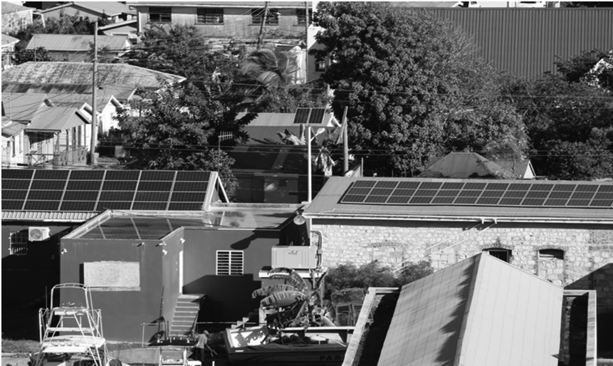
FIGURE 6.4 Solar PV installations on the island of Antigua (2018).
