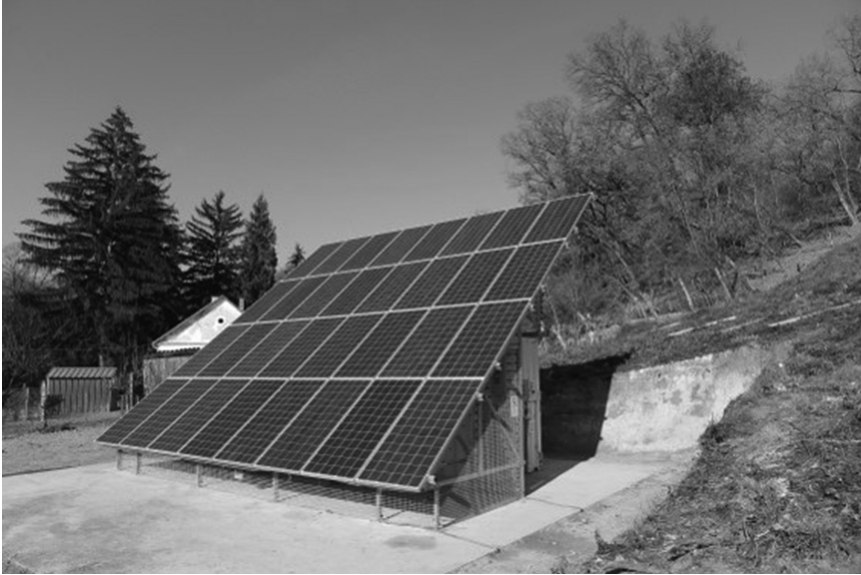
FIGURE 11.4 Container microgrid when installed [38]. (Source: E.ON, Hungary grid innovation department, 2016.)
