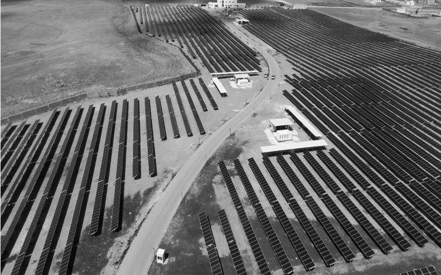
FIGURE 13.1 Grid-connected solar PV project near Amman, Jordan. (Courtesy of Mohammad Shehadeh, Philadelphia Solar.)
