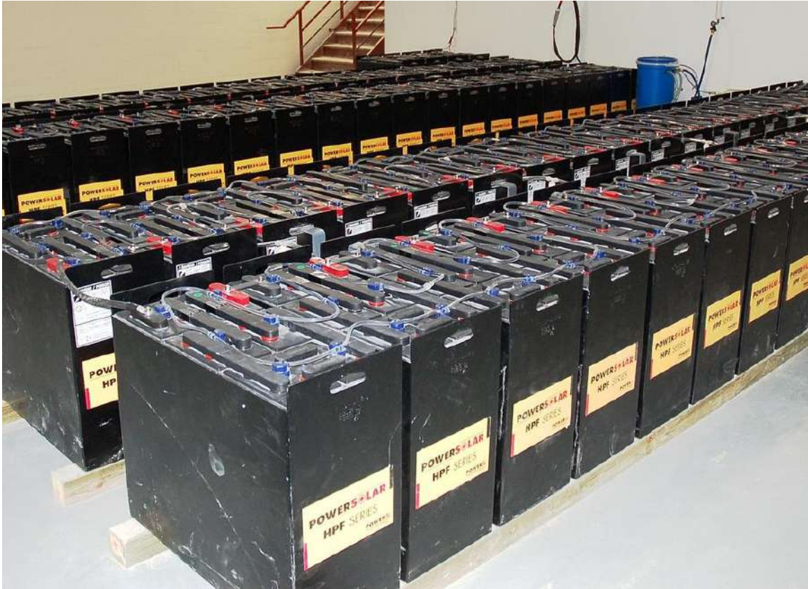
Figure 2-1. A battery array providing 60KW at 480VDC as backup for a corporate data center. (Photo by permission of Hybridyne Power Systems, Canada, Inc., and the Hybridyne group of companies. Copyright by Hybridyne, an internationally registered trademark of Hybridyne Power Systems Canada Inc. No right of further reproduction unless specifically granted by Hybridyne.)
